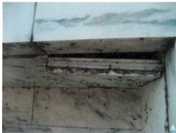
DAMAGE TO EXTERIOR OF THE HART SENATE OFFICE BUILDING.
