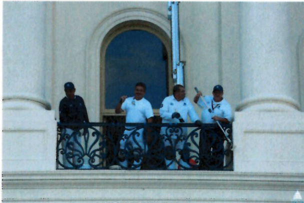
THE CAPITOL BUILDING PAINT BRANCH PUTS THE FINISHING TOUCHES ON THE SAFETY BANNISTER IN PREPARATION FOR POPE FRANCIS' VISIT.
