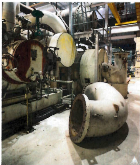
CAPITOL POWER PLANT'S AGING CHILLERS.
