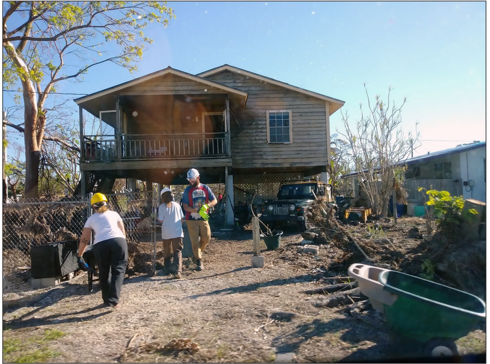
Figure 3: Nonprofit Volunteer Team Clearing Debris in Big Pine Key, Florida after Hurricane Irma
