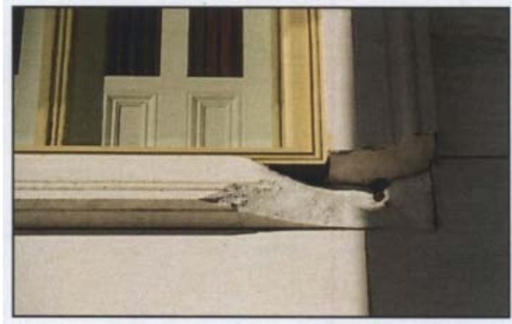
Missing stone around a Capitol Building window.
