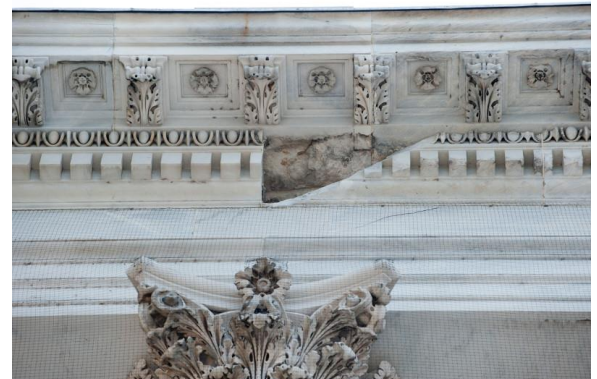
Spalling stone on the U.S. Capitol Building.
