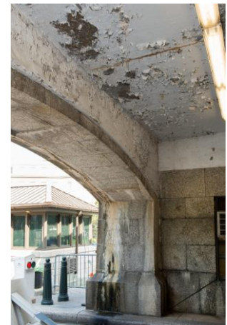
Deteriorated Senate Underground Garage.
