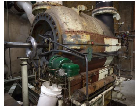
Chiller reaching the end of its life expectancy.
