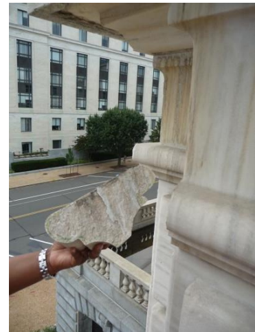
Deteriorating stone on the Russell Senate Office Building exterior.
