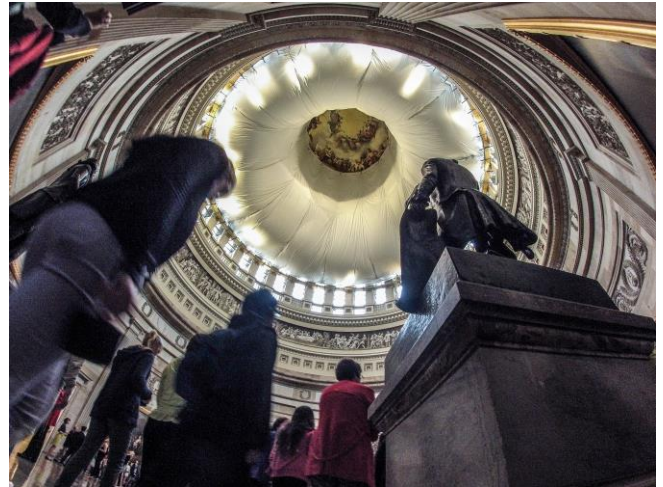
Safety canopy over the Rotunda in support of the Capitol Dome Restoration.
